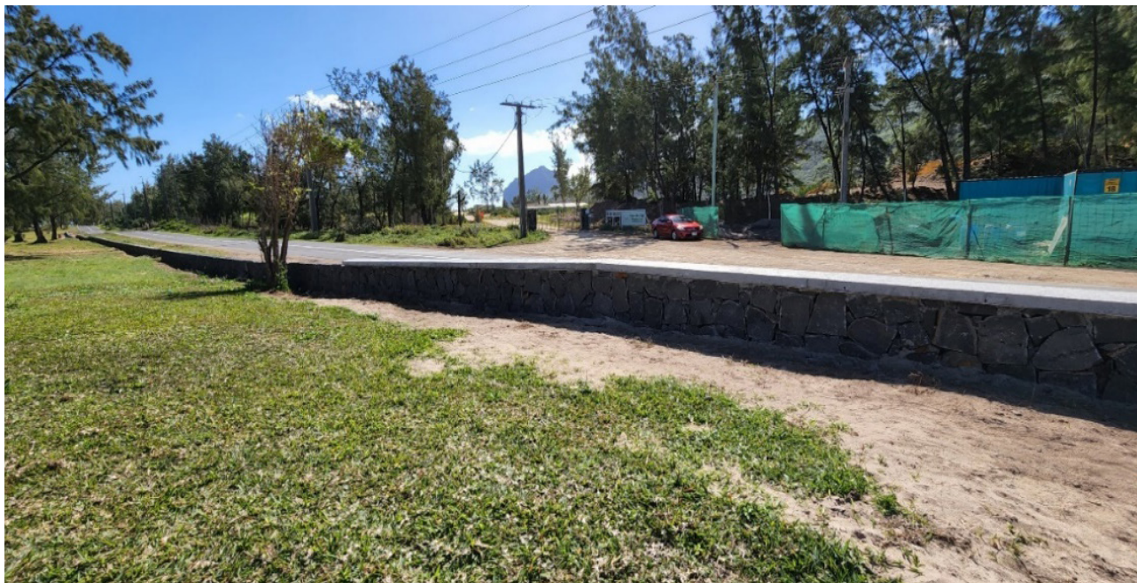
Construction of Low Stone Masonry Wall at La Prairie in context of BMP (Phase 1)
